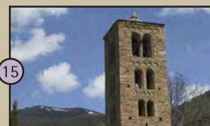
15 Belfry of Sant Martí de Bescaran: This is the only structure that remains standing from the former Romanesque church. It has quite similar to the Romanesque belfries found in the Boi valley.
